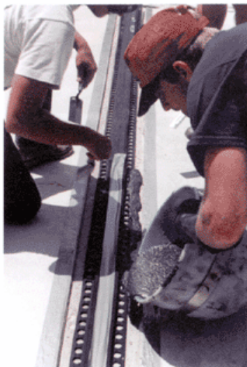
A glass-filled polyurethane nosing is poured into the joint gap to encapsulate the expansion joint flanges, or "wings." The wings on each side of the Thermaflex expansion joints provide anchoring strength as well as additional labyrinth sealing.
