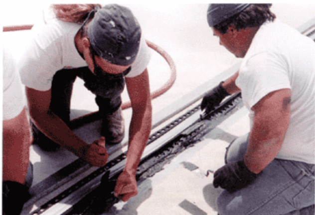
A polyurethane nosing that is quick-to-set is manually worked under, over, and around the flanges, or "wings" of the Thermaflex expansion joint system to secure it to the concrete.
