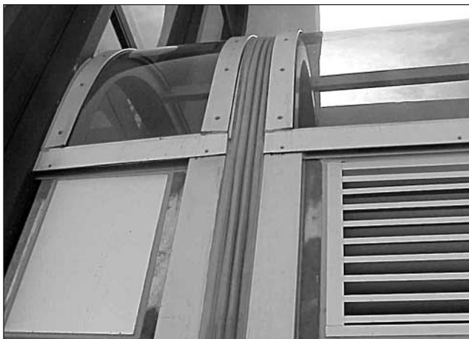
Silicone liquid-sealant and impregnated foam hybrid in hard-to-seal outside radius of skylight system.
