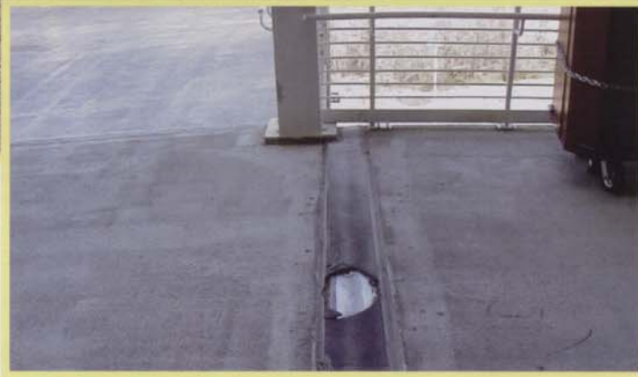
Structural materials have limitations. Cracks as the result of overstressed materials are impossible to seal and can result in dangerous structural weaknesses.
