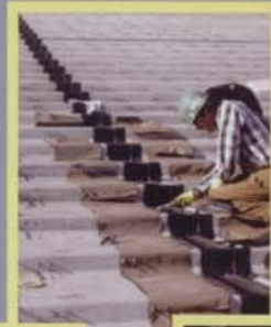
Structurally weak joints are replaced with watertight sealants to ensure safe, high-quality structures.
