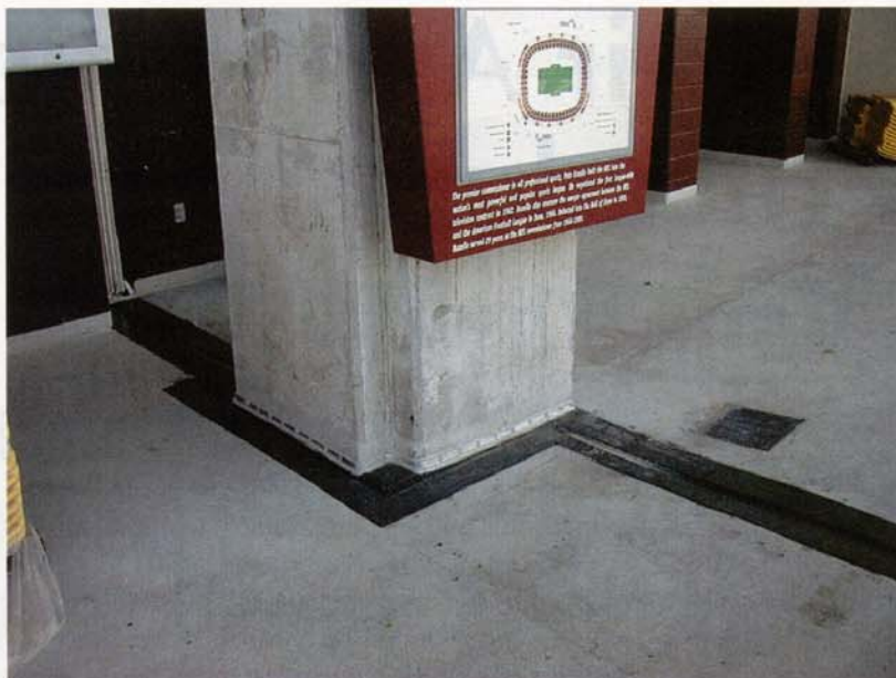
Thorough coordination between contractor and manufacturer welded joint system maintains continuity of seal around columns
