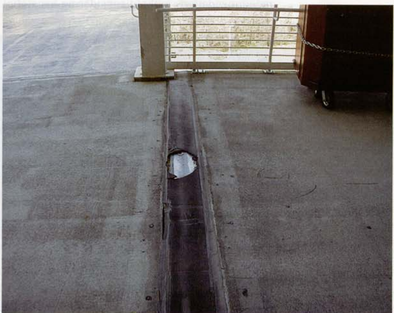
Premature failure of unsuitable joint sealing technologies can lead to hazardous conditions and costly structural deterioration
