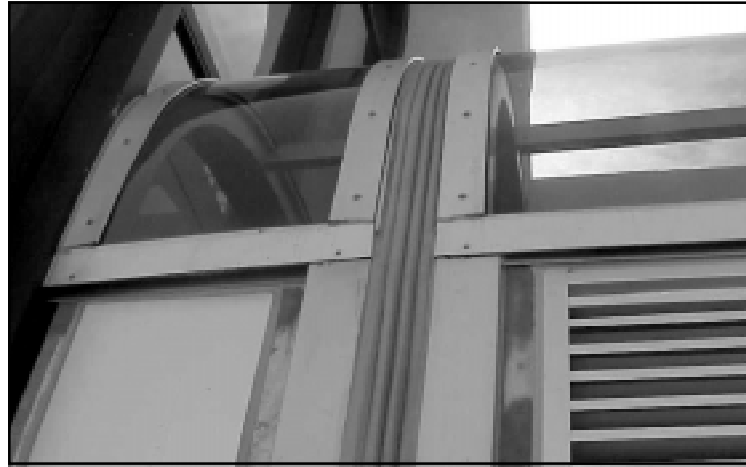
Figure 7: Silicone liquid-sealant and impregnated foam hybrid in hard-to-seal outside radius of skylight system.
